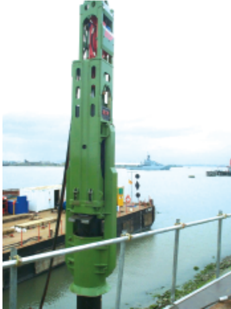
CX85, crane suspended, fitted with legs and inserts for driving steel tubular piles
